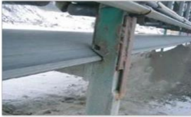
Figure-1: Structure Damage
